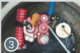
Regular Unleaded With Sump-Dri Installed
